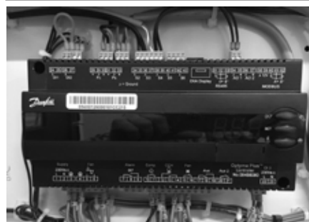
Picture 3 : Normal wiring
