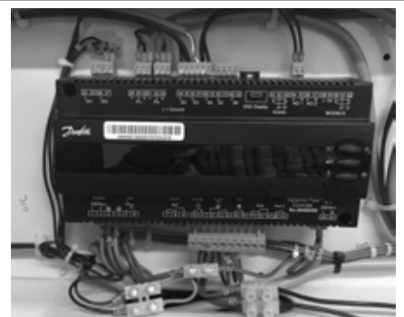
Picture 4 : Temporary wiring
